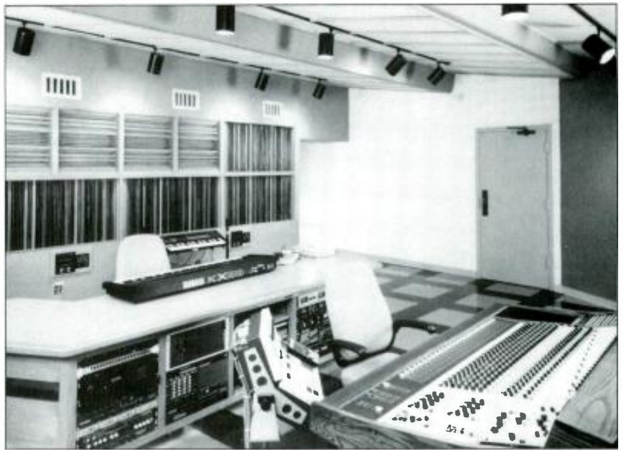
Figure 2. The control room.
