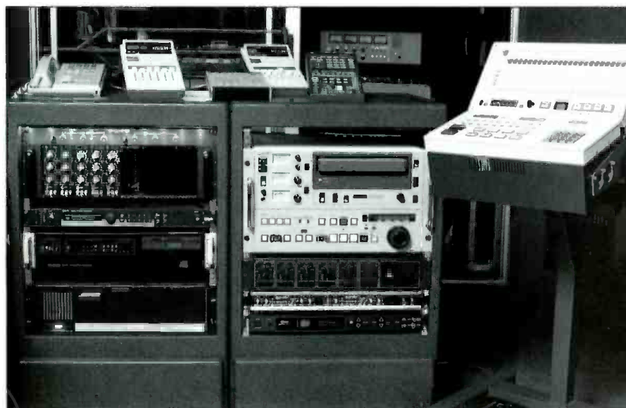
Figure 3. Critical effects/processing, video editing and auto locators are all within comfortable reach from the console position.
