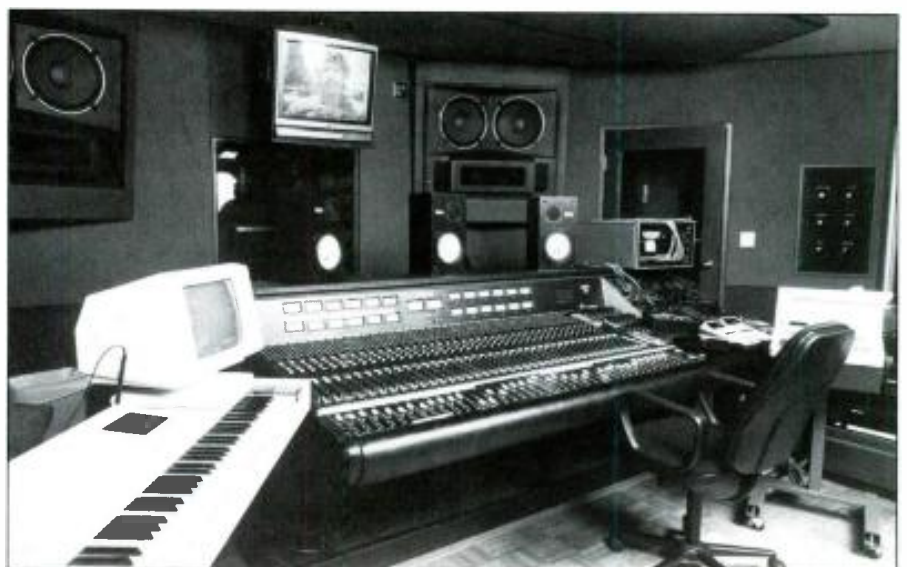
Figure 1. The control room includes a Fairlight System III and Trident console. Note the strategically-placed, centered near-field monitor.
